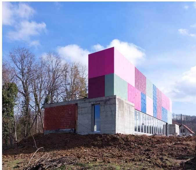
Project in Gradačac, Bosnia and Herzegovina Photo of the construction progress, February 2022
